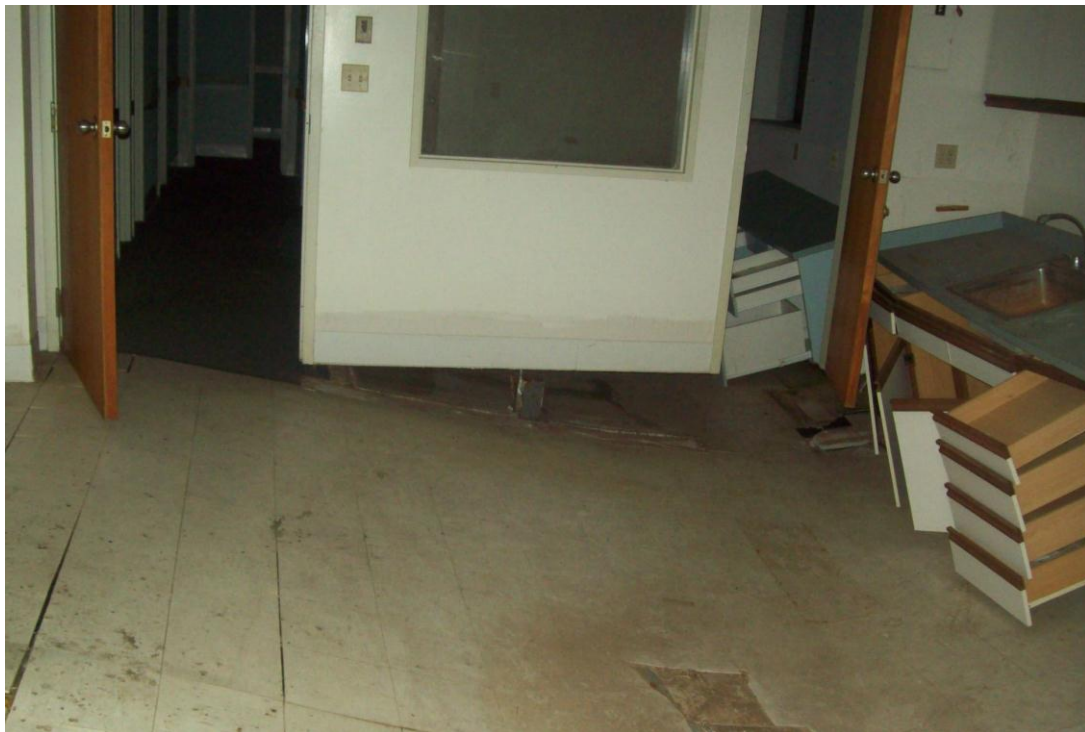
Photo 6: Floor Failure in Wing D
