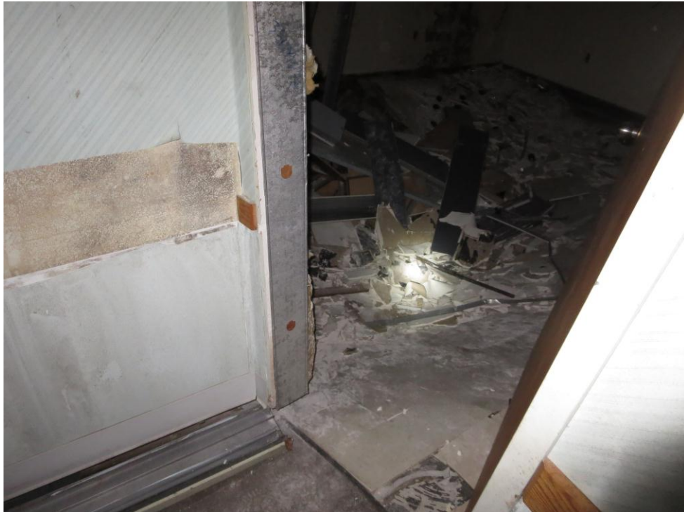
Photo 2: Floor Collapse in Wing A
