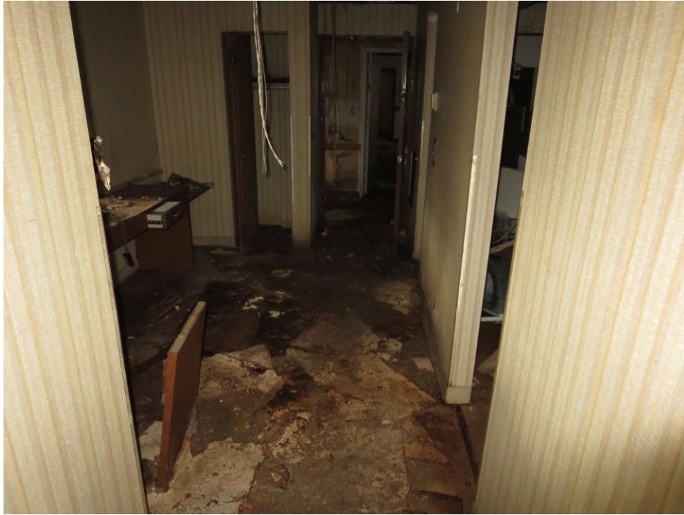
Photo 5: Water Damage / Deterioration in Wing C
