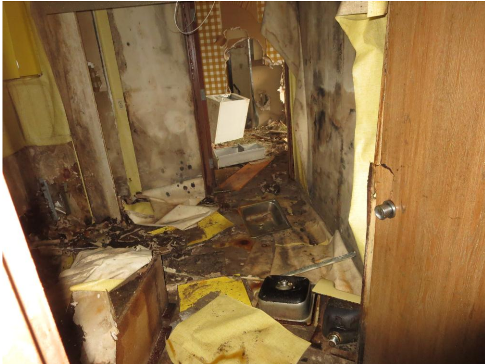
Photo 4: Fourth Floor of Wing B – Substantial Water Damage
