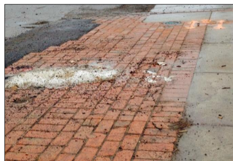
FIGURE 3: DETERIORATING STREETSAPES W. MAIN
